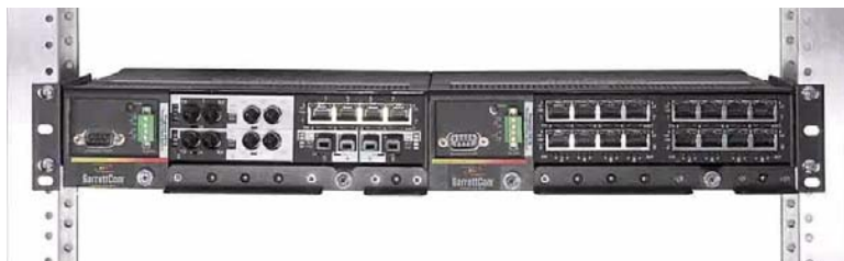
Fig 3.3.2b- Two Magnum 6K16s deployed over a K16-2Tray side-by-side to provide larger port density of 32 ports.
